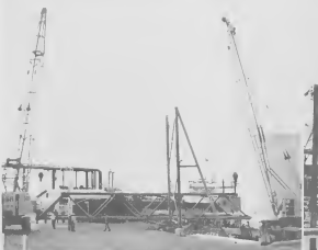
CRANES LIFTED in unison from extreme ends of the bridge. The structure will carry sixteen pipelines across the main refinery road. The pipe system will be used in connection with No. 3 Finger Pier, currently under construction. The bridge was fabricated by the Curaçao Drydock Company as part of its contract work on the finger pier. Into the structure went 1300 feet of pipe of various diameters.
